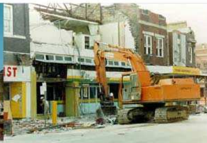
Extensive damage occurred at Beaumont Street, Hamilton.
