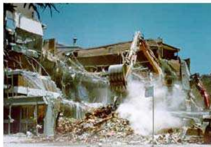
The Newcastle Workers Club was the scene of 9 deaths and many injuries when it collapsed.
